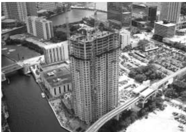
New developments – such as Brickell On the River, in the "lower river" – include public riverwalks to link the greenways on the river's banks.
