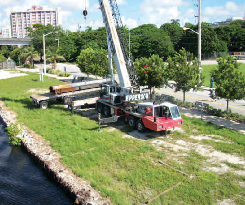
Miami River Voluntary Improvement Program (VIP) item being addressed via replacing deteriorated seawall.
